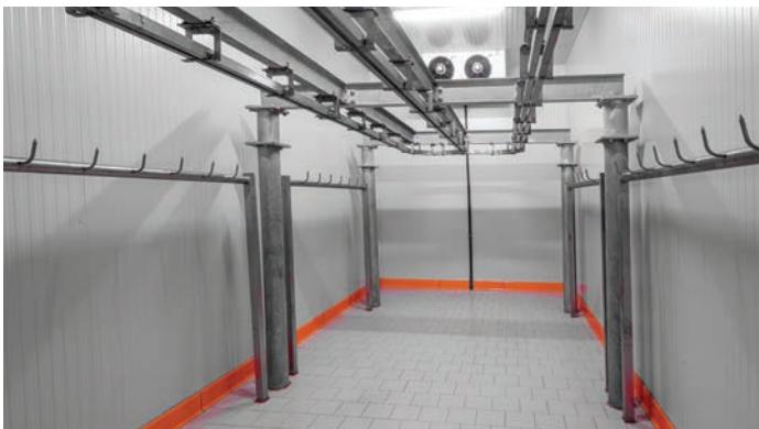
Cold Room and Storage
