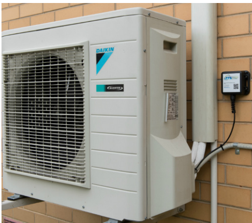
DRED enables control of existing A/C systems
